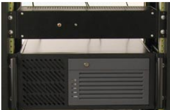
POES Station and Tracking Controller
